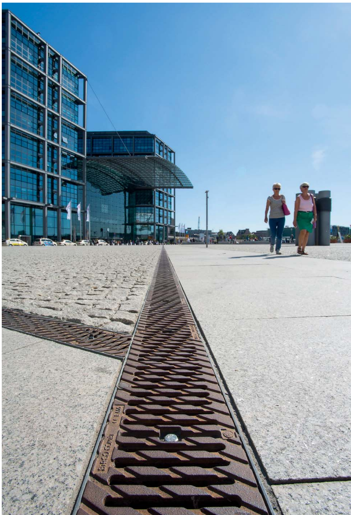
BIRCOLight op Washingtonplatz in Berlin
